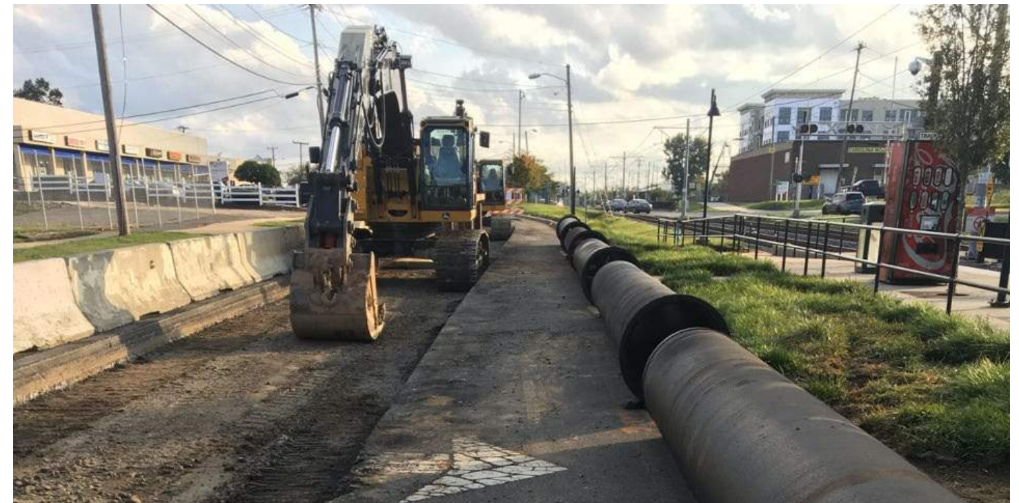
Infrastructure is critical to growth and requires long-term planning based on community-driven land use policies. (Image source: www.charlottenc.gov)
