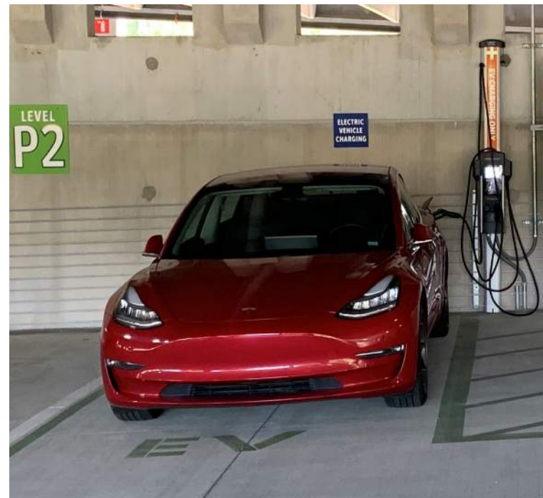
EV Designated Parking Spot in a Parking Deck. (Image source: VHB)
